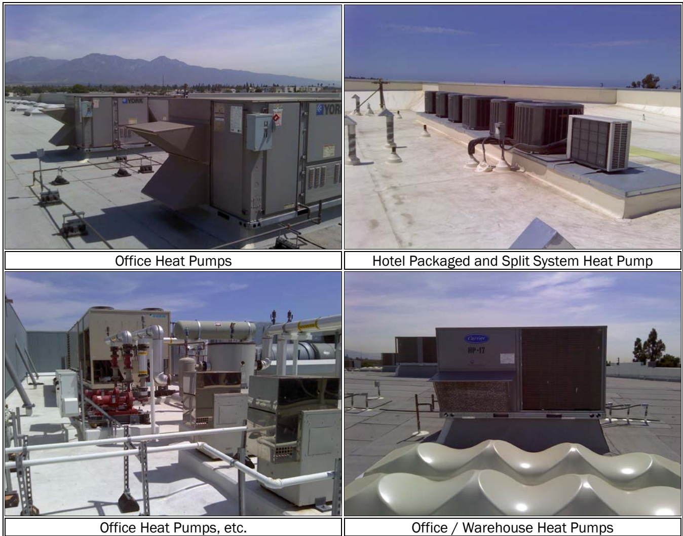
Figure 27: New Construction Rooftop Examples
