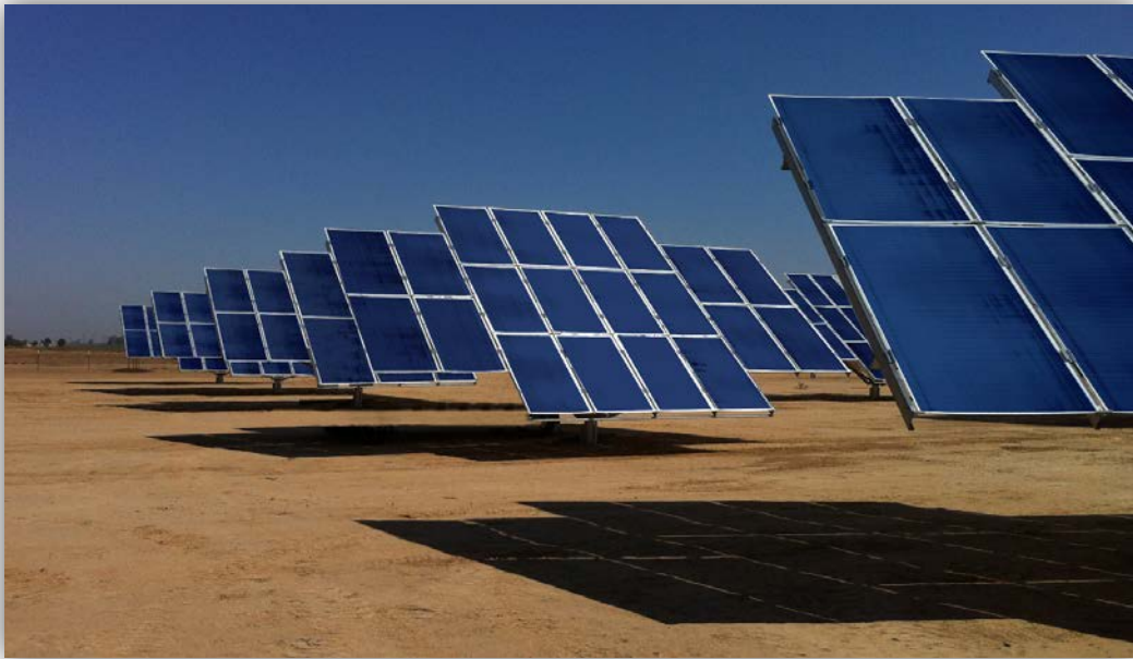
Figure 20: Project featuring Solaria modules for the City of Atwater, CA
